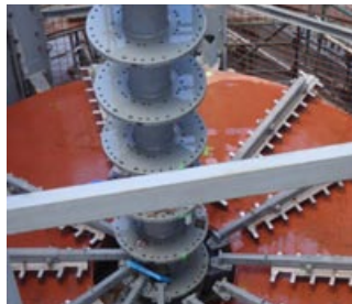
Inside a drying tank
