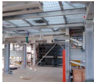
Silo discharge conveyors
