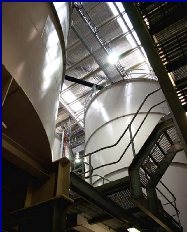
Storage silos used for the incoming biosolids
