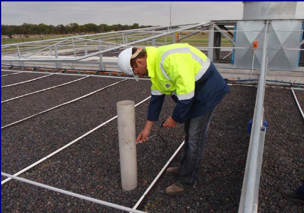
Pre-commissioning of the biofilter
