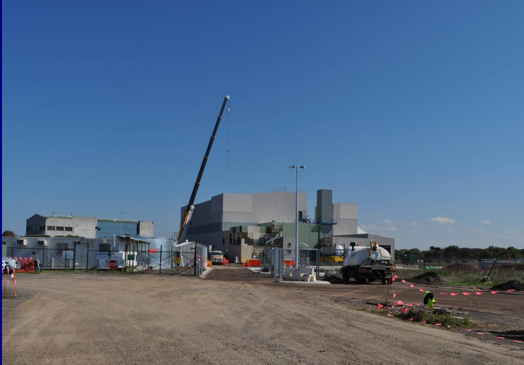
Front view of the Biosolids Treatment Facility
