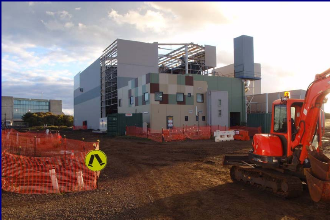
Front view of the Biosolids Drying Facility as cladding is fitted and equipment is installed.
