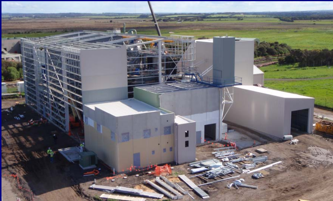
Aerial view of the front of the Biosolids Drying Facility as cladding is fitted and buildings are painted.
